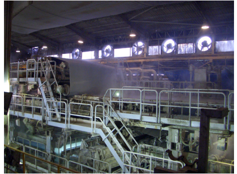
Forming section of the board machine at Barcelona Mill
