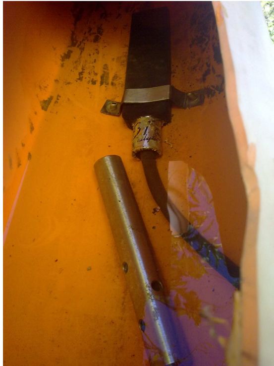
Fig. 15: particular of the area-velocity probe and the intake suction device for the monitoring station” Varese IN”
