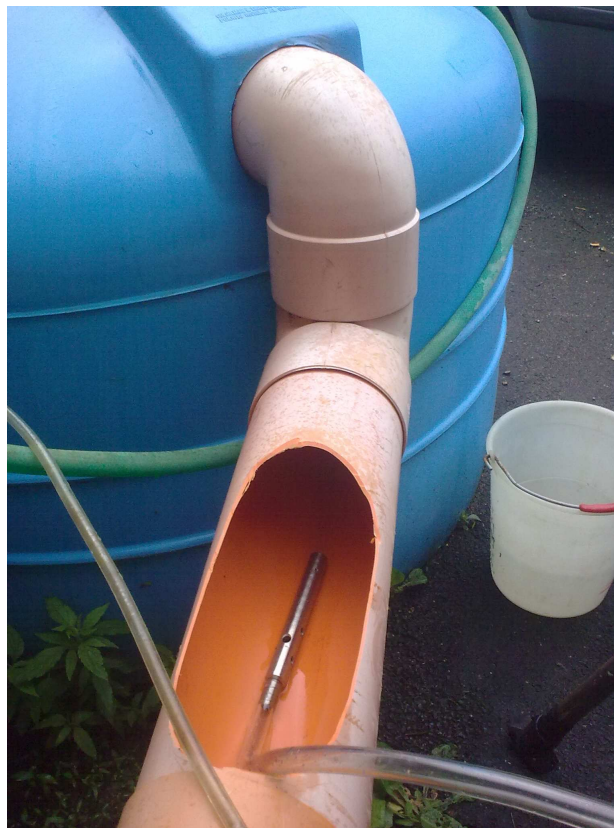
Fig. 18: installation of the intake suction line into for the monitoring station” Varese OUT”
