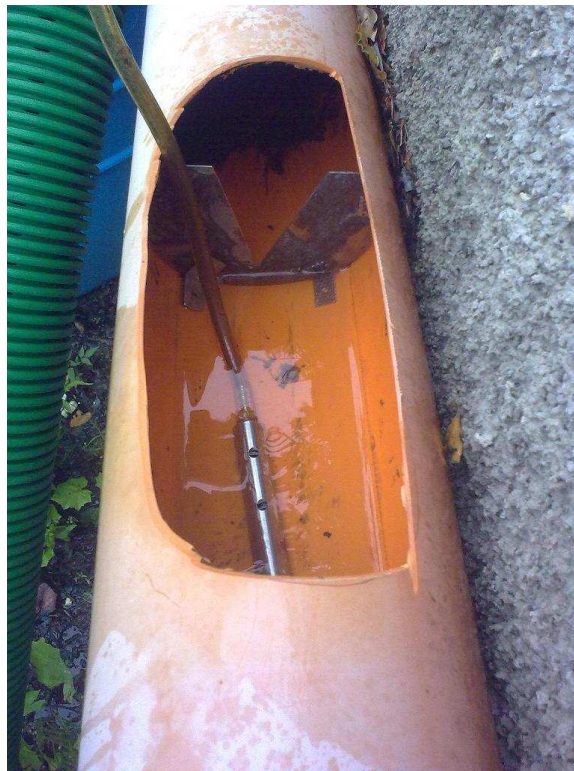
Fig. 16: installation of the intake suction line for the monitoring station” Varese IN”
