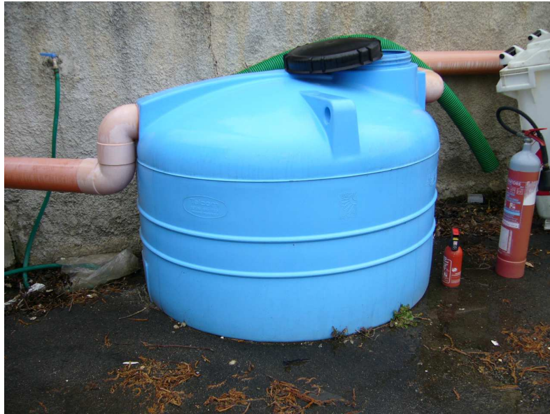
Fig. 13: particular of the existing treatment system
